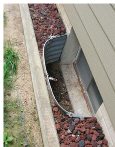
An unprotected window well.
