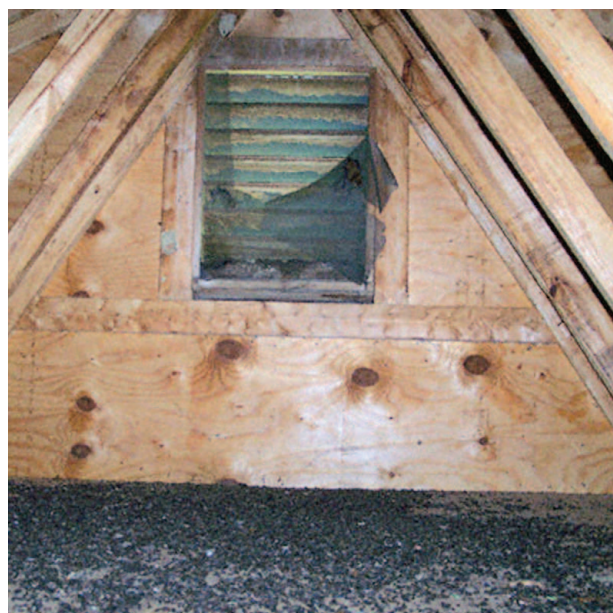
Bat guano in attic with damaged screen.
